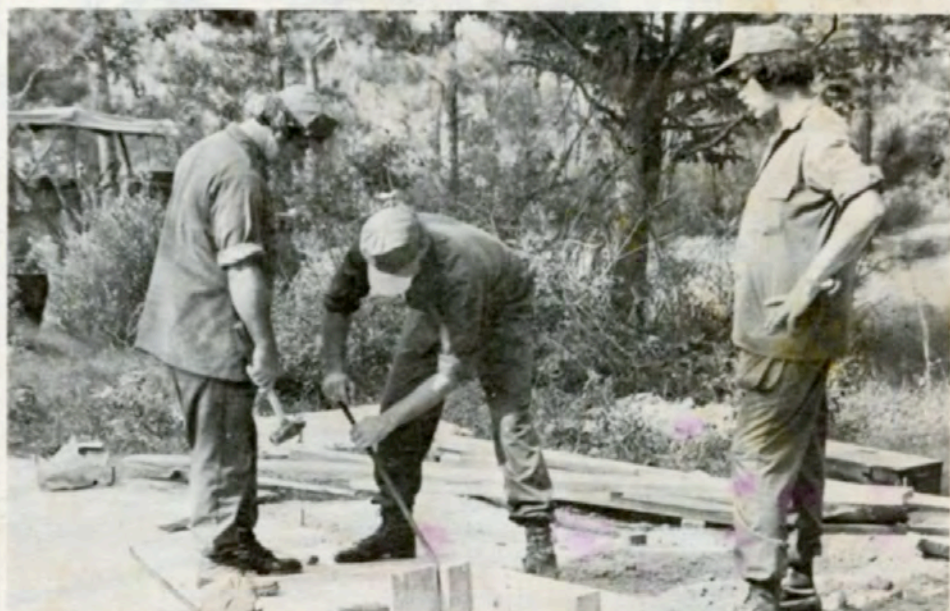
GETTING READY ON THE OUTSIDE. . . National Guard members work under the hot Louisiana sun as they build new facilities at Camp Beauregard.
