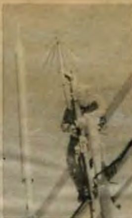
CMS Charles R. Nastasia connects coaxial cable to an antenna installed atop Highland Peak Nevada.
