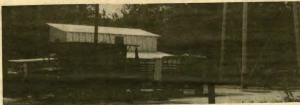
Equipment and manpower donated by the 528th Engr Bn helped to restore water to Georgetown after a series of water systems plague the town. (LaARNG Photo)
