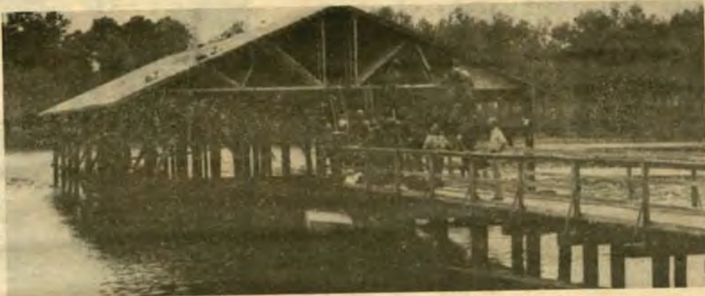
Members of the 527th Engr Bn work on a 32-slip boat marina for the Cypress-Black Bayou Recreation and Water Conservation District. (LaARNG Photo)
