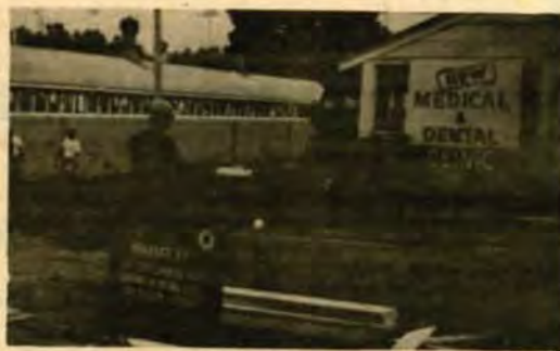
Several members of the 159th CES participate in excavation and construction for the Medical and Dental Facility at the ANG Training Site, Alpena, MI.
