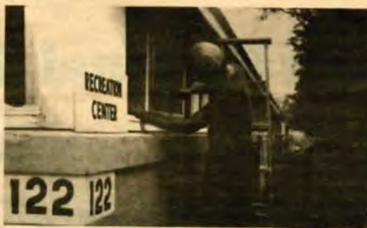
SSgt Norris (left) and SSgt Jackson make repairs to the Recreation Center Facility at the ANG Training Site, Alpena, MI.
