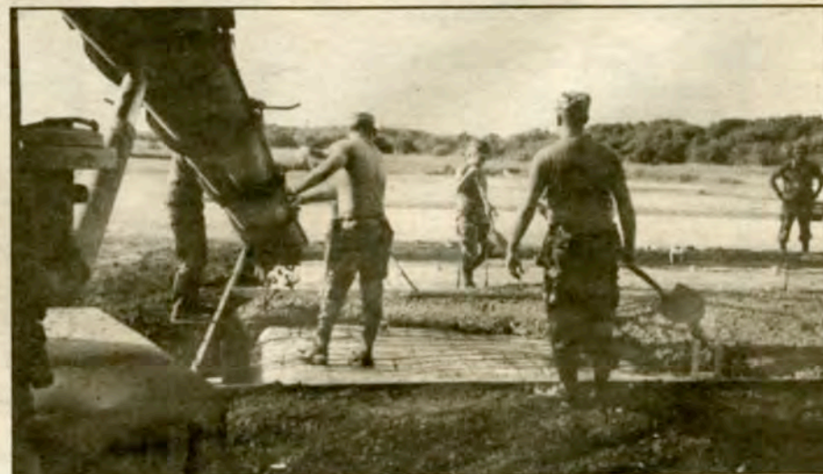
Members of Charlie Company, 205th Engineer Battalion pour a concrete slab, one more step towards a 24' x 40' dining pavilion, at Fort Sill, Okla. (Photo by 2LT Paul Treadway, 205th ENGR BN)
