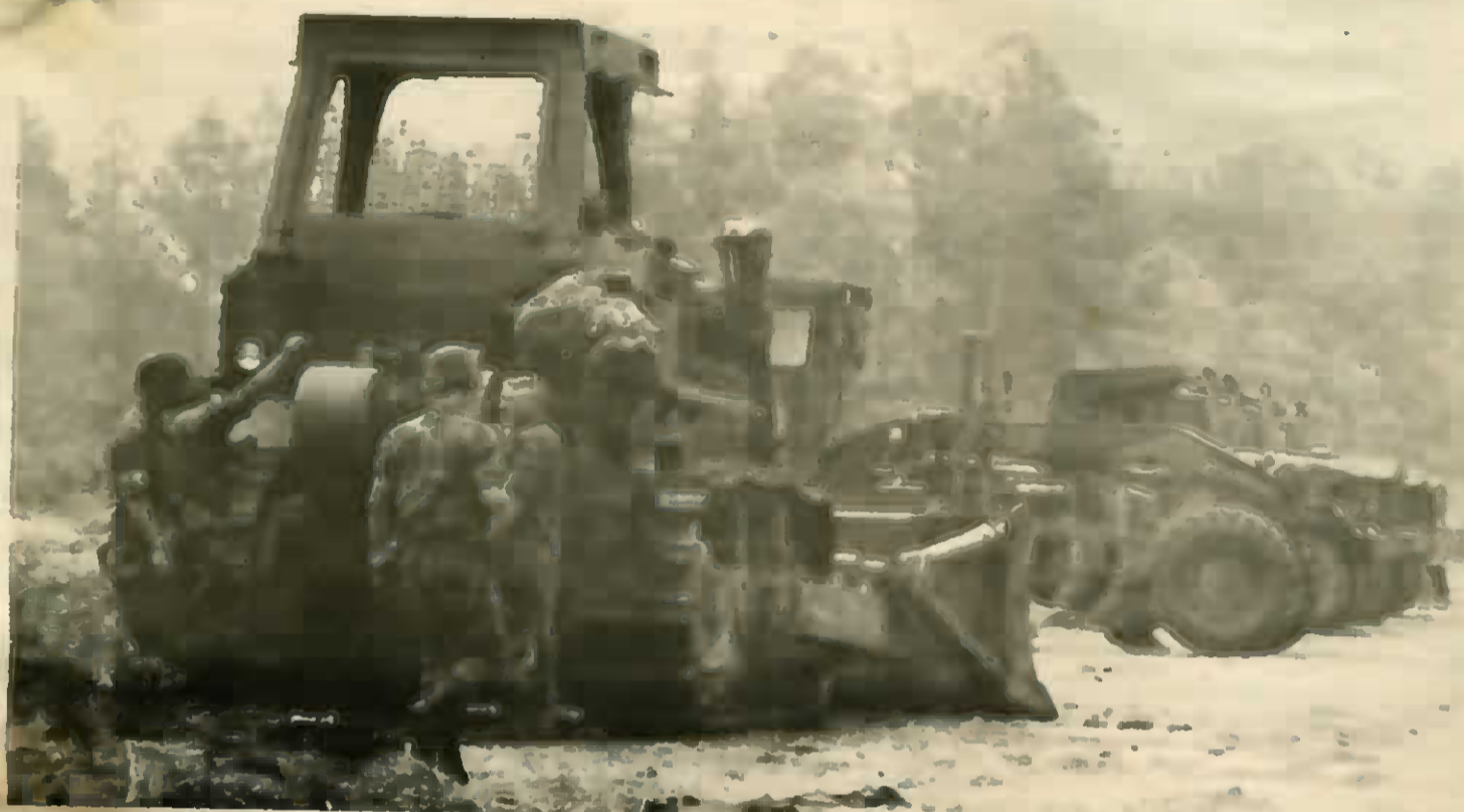
Company A, 769th Engr. Bn perform maintenance on horizontal equipment during construction efforts across the state.
