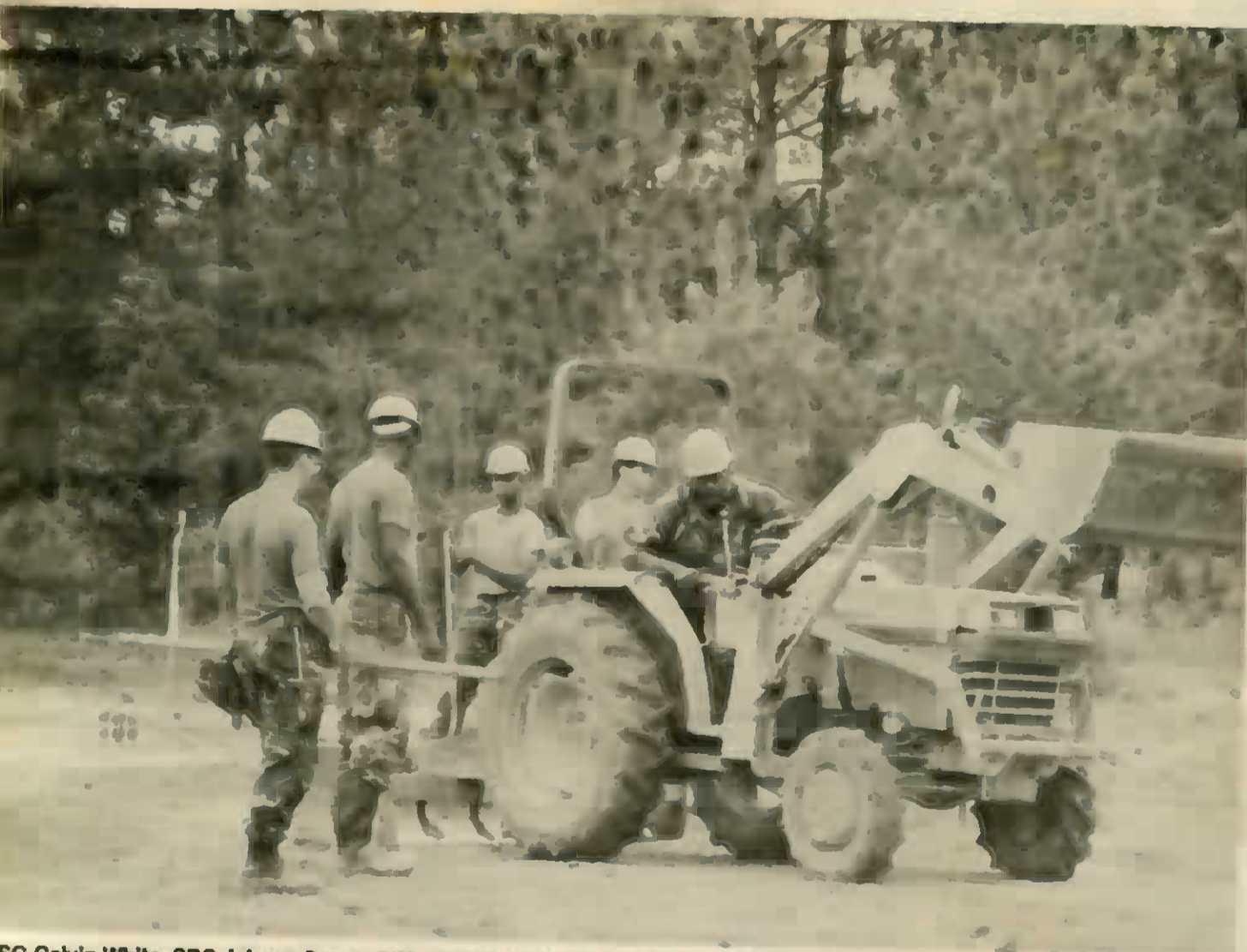
SSG Calvin White, SPC Johnny Green, PFC Jonathan Martin and SSG Grandison Garnett work to level the grade of the slab.
