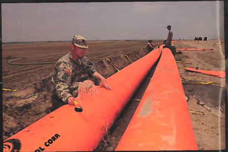
GRAND ISLE, La. – Soldiers with the Louisiana Army National Guard pump water into a Tiger Dam interlocking water diversion system in Grand Isle, La., May 29, 2010, in support of the Deepwater Horizon oil spill cleanup efforts. Photo: Staff Sgt. Jeffrey T. Barone
