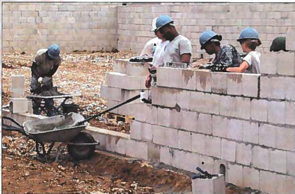
Soldiers from the 225th Engineer Brigade lay blocks July 15, 2010, in a mock village used to train multinational troops who are preparing to deploy overseas. The Louisiana Army National Guard has been supporting this training effort by providing rotational engineer expertise and assets for the Joint Multinational Readiness Center in Hohenfels for the past several years.
